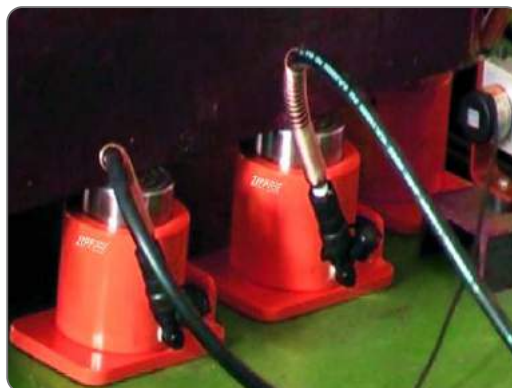
ZRSCS-502 Rapid transit system Synchronous Lift application
